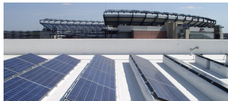
Solar cell panels near Gillette Stadium in Foxborough, Mass.
